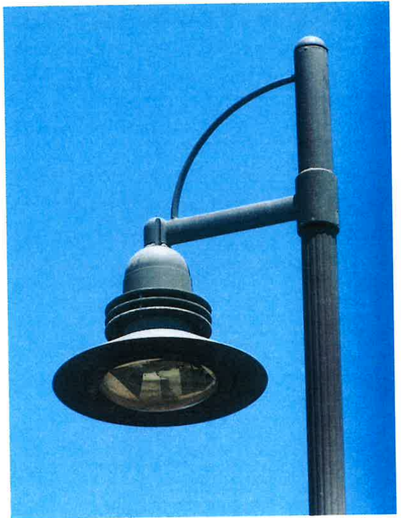
Closeup of Fixture and Pole Arm
