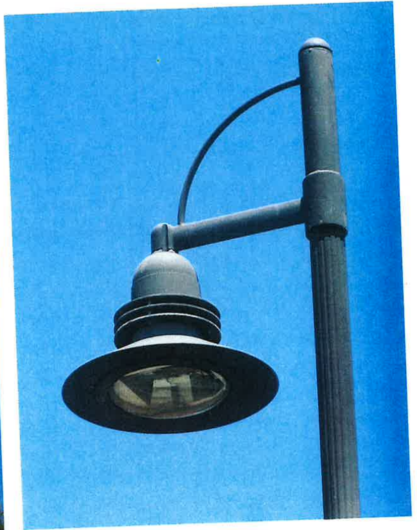
Closeup of Fixture and Pole Arm
