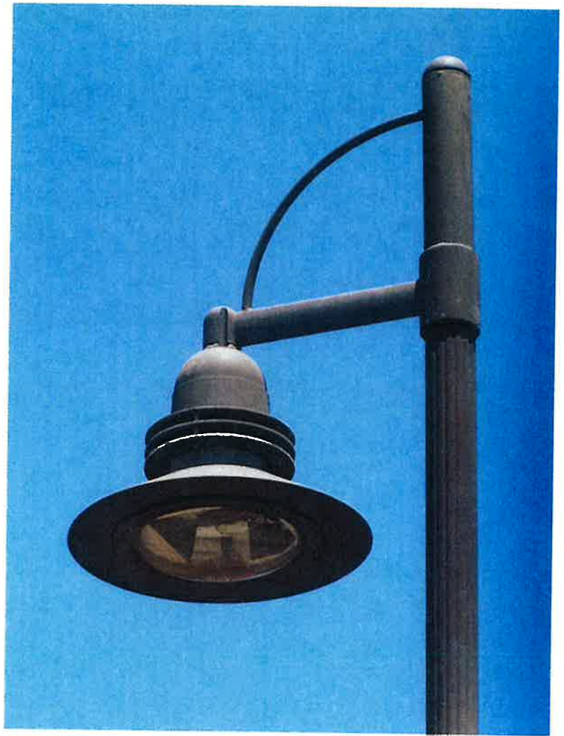
Closeup of Fixture and Pole Arm
