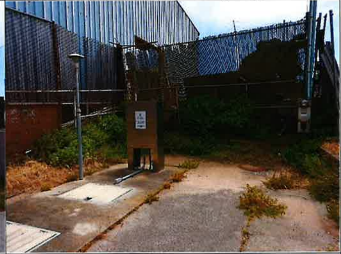
Lift Station Equipment
