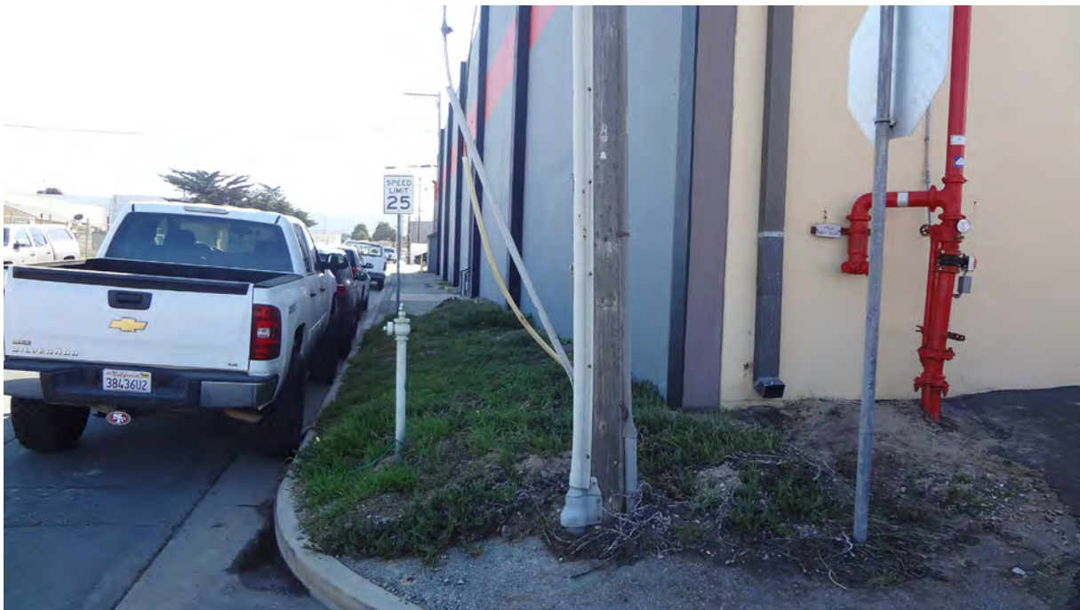
Photo F3: This photograph shows the lack of wheelchair ramps and the lack of complete sidewalks at the southeast intersection of Catalina Street and Ortiz Avenue. The City has preliminary draft public improvement plans to rectify this as part of its Stormwater Proposition 1 Grant endeavors.
