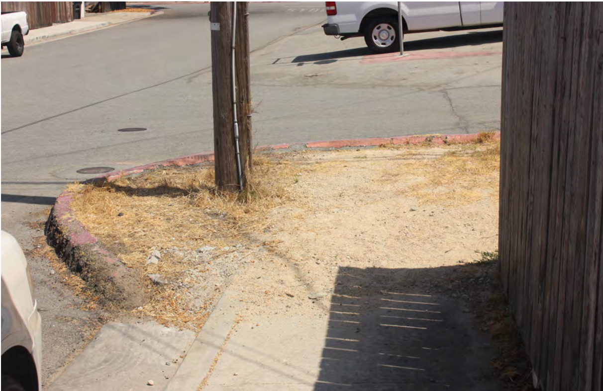
Photo F11: This photograph shows the missing sidewalk and ramp at the southeast corner of the Holly Street and Dias Avenue intersection.
