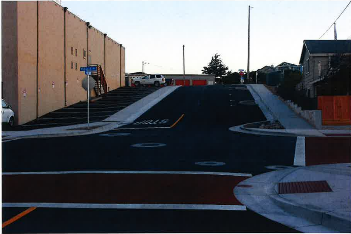
Photo F8: This photograph is taken at the Redwood Avenue and Hickory Street intersection, looking north towards the City Hall, and shows how the grade of Hickory Street is too steep for wheelchair access. This block was recently rebuilt to add sidewalks on the right side, but the grade and narrow right-of-way precluded attaining a slope suitable for wheelchairs.
