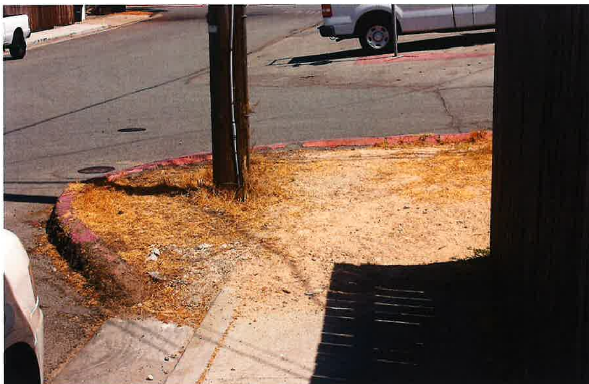
Photo F11: This photograph shows the missing sidewalk and ramp at the southeast corner of the Holly Street and Dias Avenue intersection.
