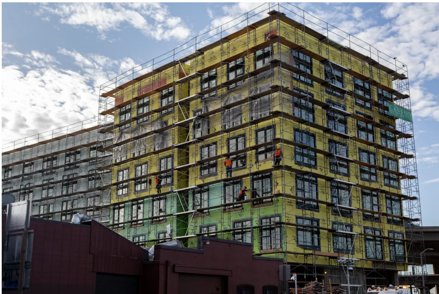
A Factory OS pre-fab apartment building in West Oakland. Photo by Anne Wernikoff for CalMatters
