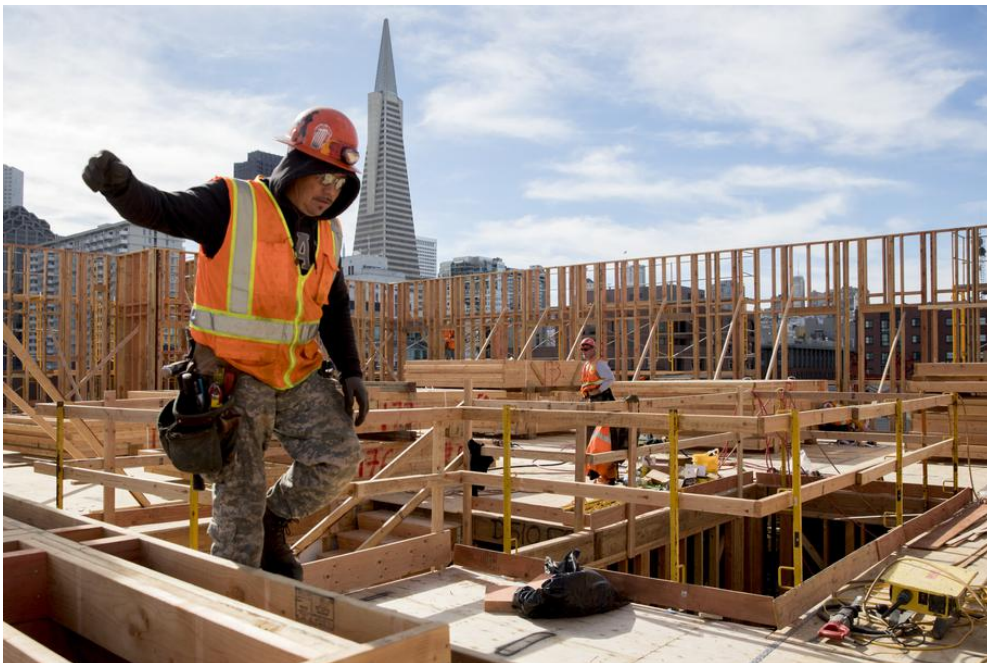
Workers construct two affordable housing developments, one for seniors and one for multi-family use, on the Embarcadero near Broadway in San Francisco in 2020.
