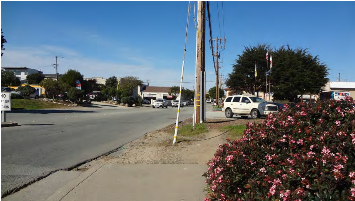
Photo F2: This photograph is taken from Contra Costa Street upon entering Sand City from Del Monte Avenue, and shows the lack of sidewalk within the railroad corridor. Both sides of Contra Costa Street are missing sidewalks in this area.
