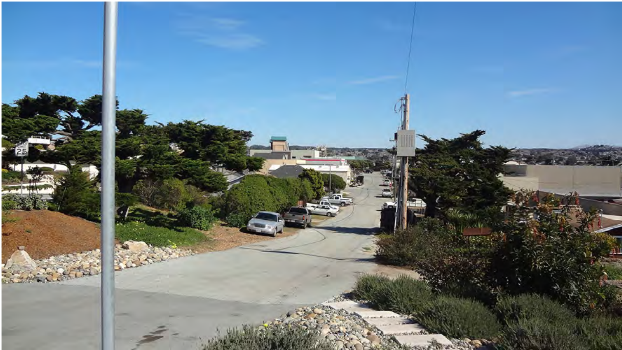
Photo F8: This photograph is taken at the Redwood Avenue and Hickory Street intersection, looking north towards the City Hall, and shows how the grade of Hickory Street is too steep for wheelchair access. This block was recently rebuilt to add sidewalks on the right side, but the grade and narrow right-of-way precluded attaining a slope suitable for wheelchairs.
