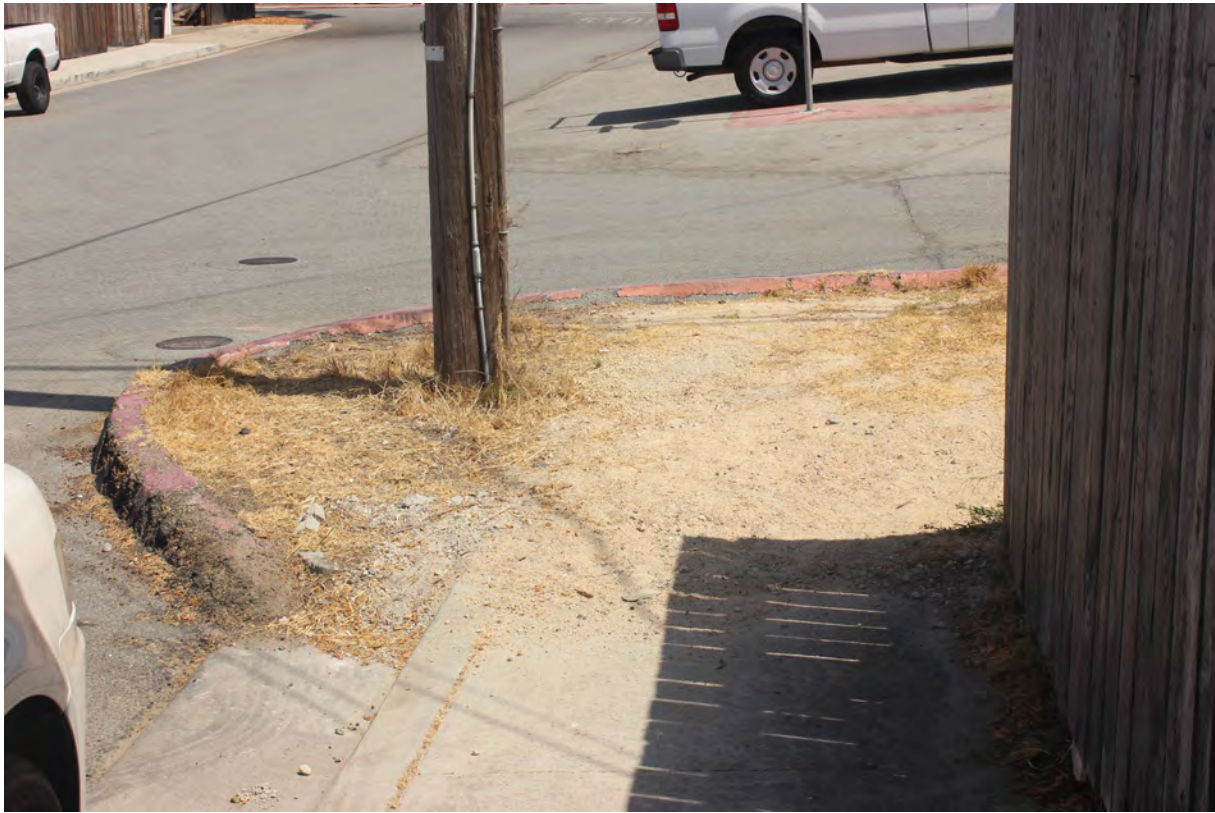
Photo F11: This photograph shows the missing sidewalk and ramp at the southeast corner of the Holly Street and Dias Street intersection.
