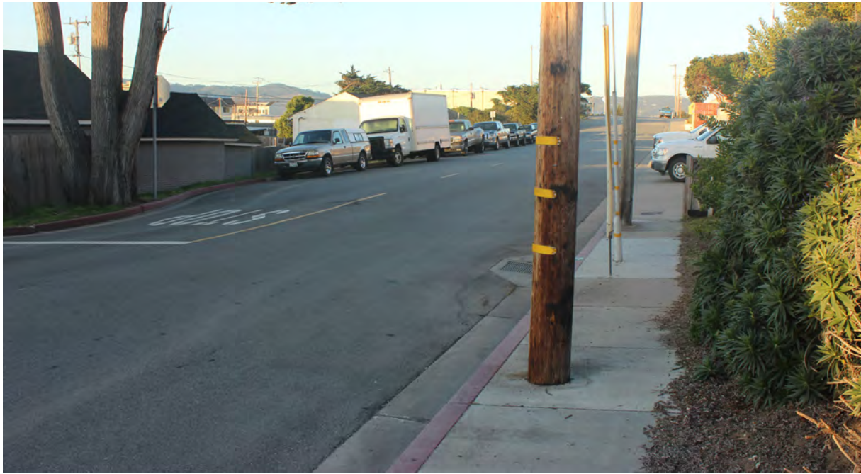
Photo F10: This photograph is taken at the corner of California Street and Holly Street and shows the lack of sidewalks and wheelchair ramp.
