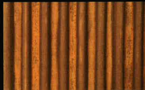
CORRUGATED RUSTED METAL PANEL
