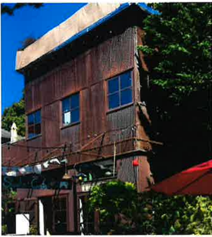
CORRUGATED METAL RUSTED BY THE SEA AIR
