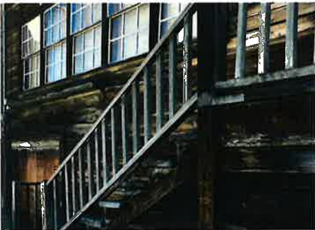
WOOD WEATHERED BY THE COASTAL ENVIRONMENT
